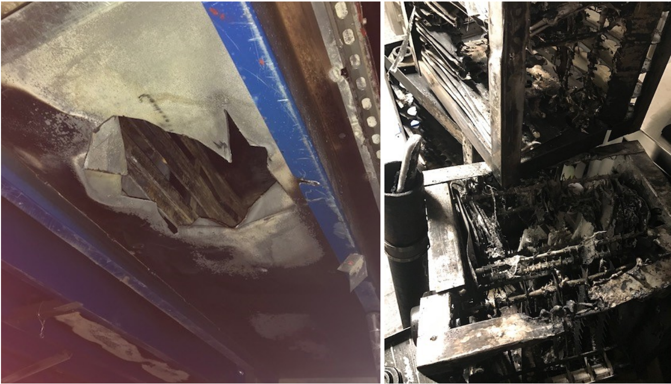
Shown above: Fire department access holes made in the ESP (left) and damaged ESP cells (right).
